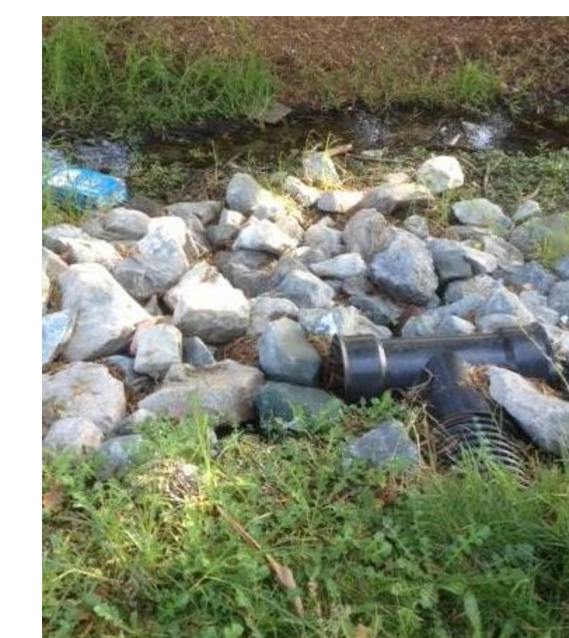
A drainage pipe, Peralta Creek Site 2.
